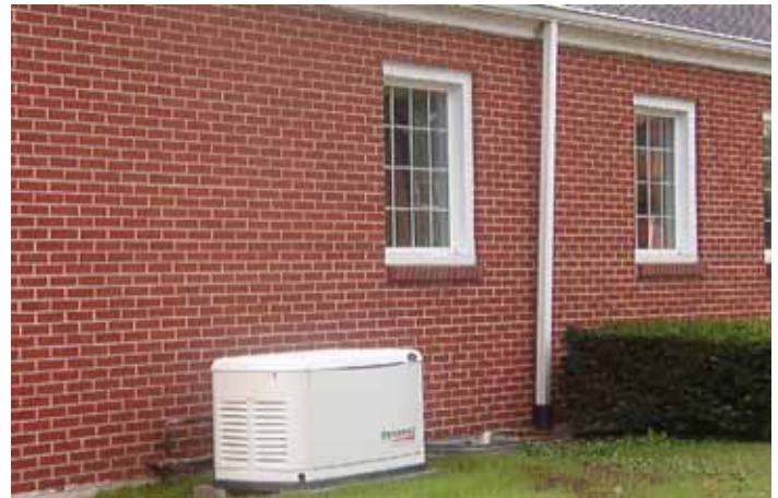
Pictured above our new generator and windows.
